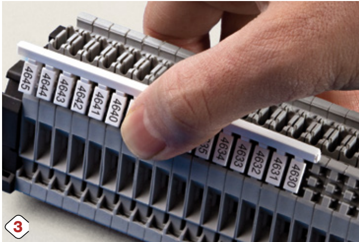
3 Insert the tags directly into the terminal block series using light pressure.
